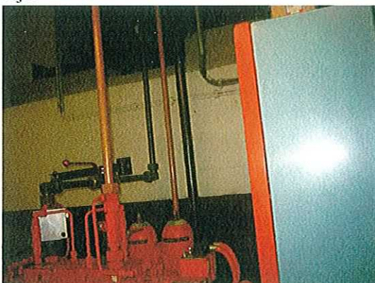
Hydraulikkaggregat i lukehus Opstveitvatnet. Oljeinnhold ca. 100 liter.
