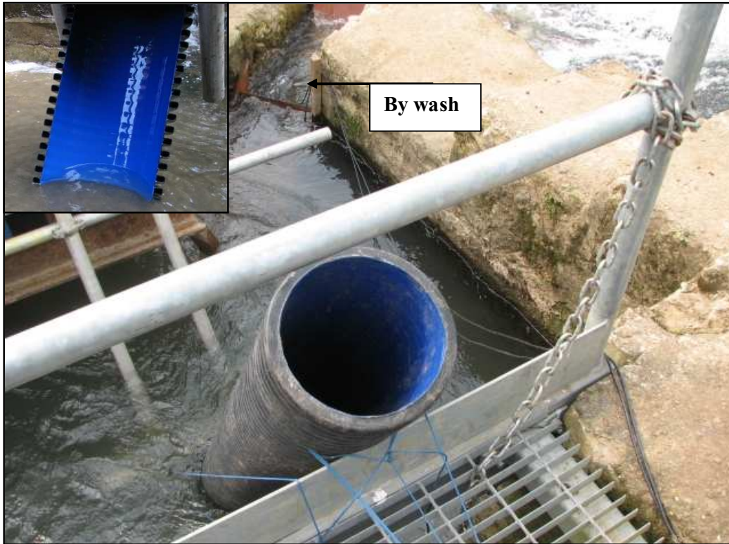
Figure 2: photo showing the pipe used to introduce fish to the intake area above the turbine and by-wash, and the escape window at the end of the pipe (inset).
