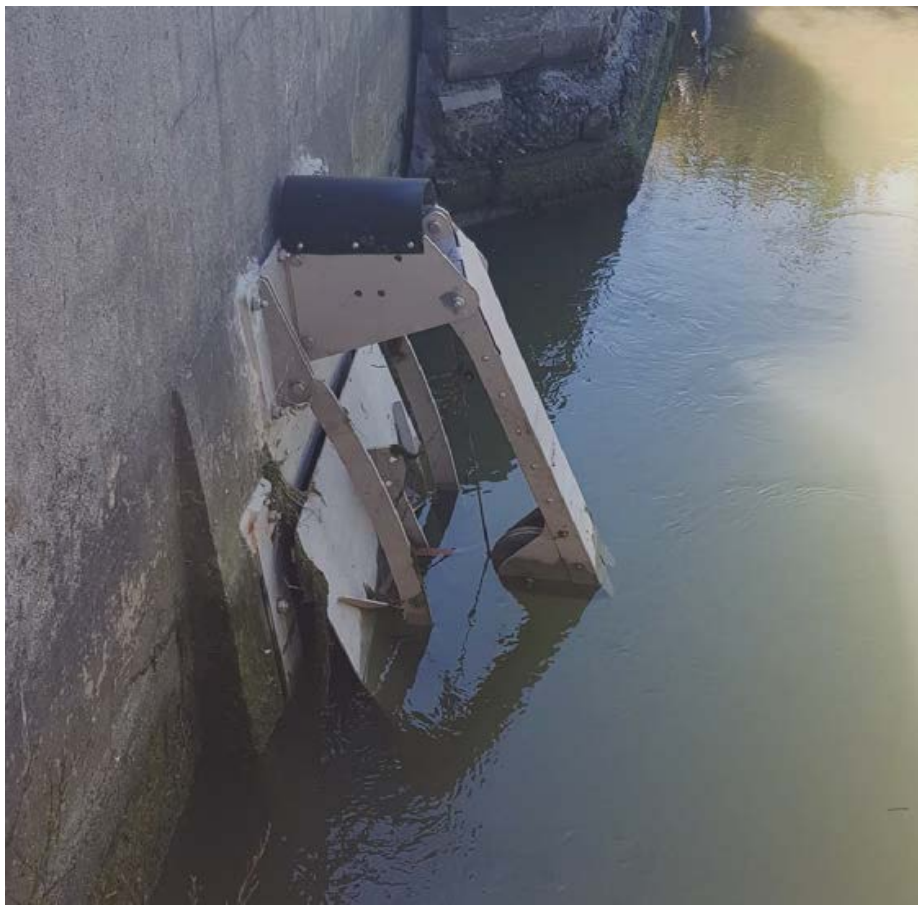
Figure 5-12: A tide gate retrofitted with a fish friendly counter weight system in Christchurch. Credit: Paul Franklin.
