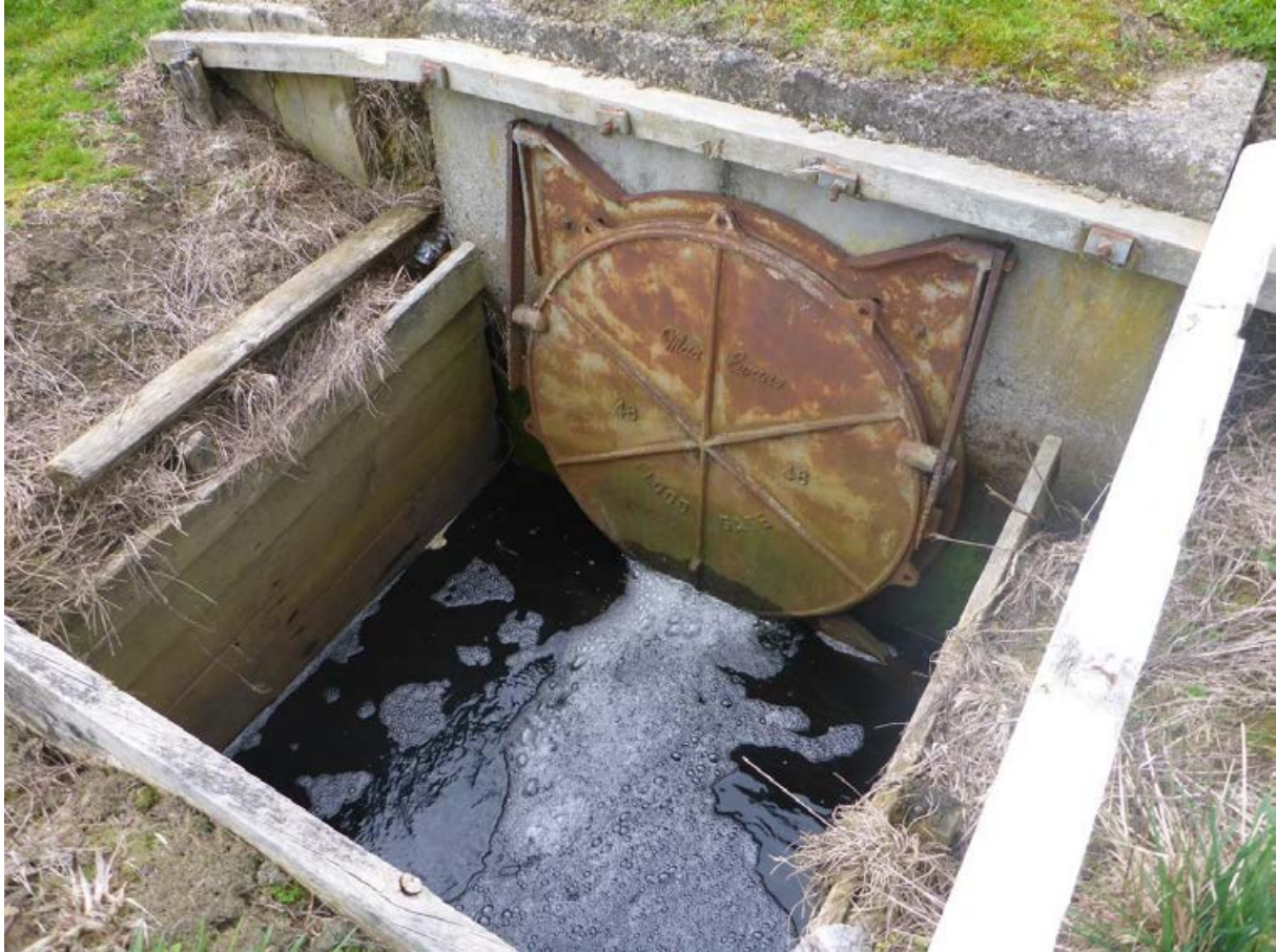
Figure E-8: An example of a tide gate from the Waikato River catchment. Credit: Rimutere Wharakura.
