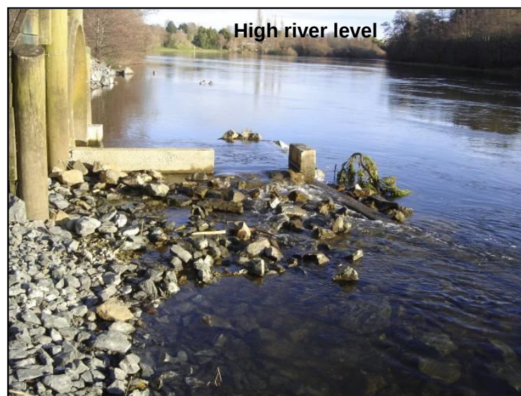
Figure 5-2: Example of a concrete rock ramp below a culvert that is oriented perpendicular to the downstream water body. A receiving pool has been added to the base of the culvert to direct the ramp downstream along the river margin. This provides the foundations for a low gradient sloping ramp.
