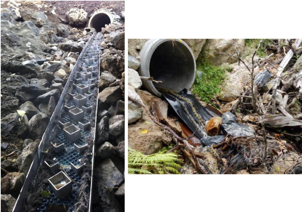
Figure 8-1: Examples of novel fish passage remediation solutions for perched culverts. Left: An example of a novel fish ladder design. Right: Conveyor belt rubber being used as a fish ramp alongside mussel spat ropes.
