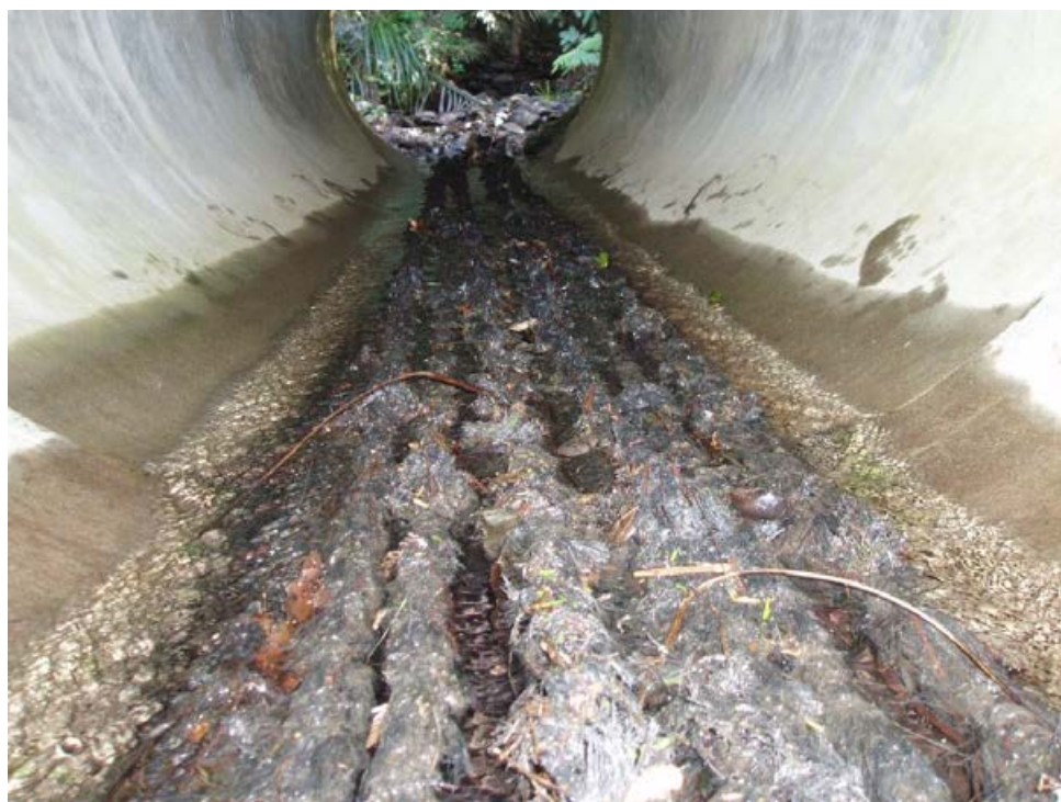
Figure 5-10: Example of good mussel spat rope installation showing fish 'swimming lanes' between ropes. Note that the number of ropes has been scaled up to match the size of the culvert. Photo: Bruno David.
