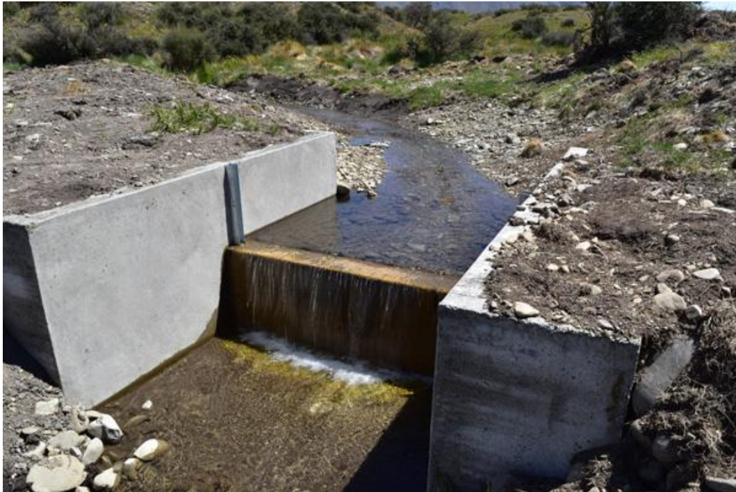
Figure 6-3: Built barrier installed in Cabbage Tree Gully, Canterbury. The barrier was built to prevent trout accessing a key lowland longjaw galaxias stronghold in the lower Waitaki River, Canterbury. Credit: Peter Ravenscroft.
