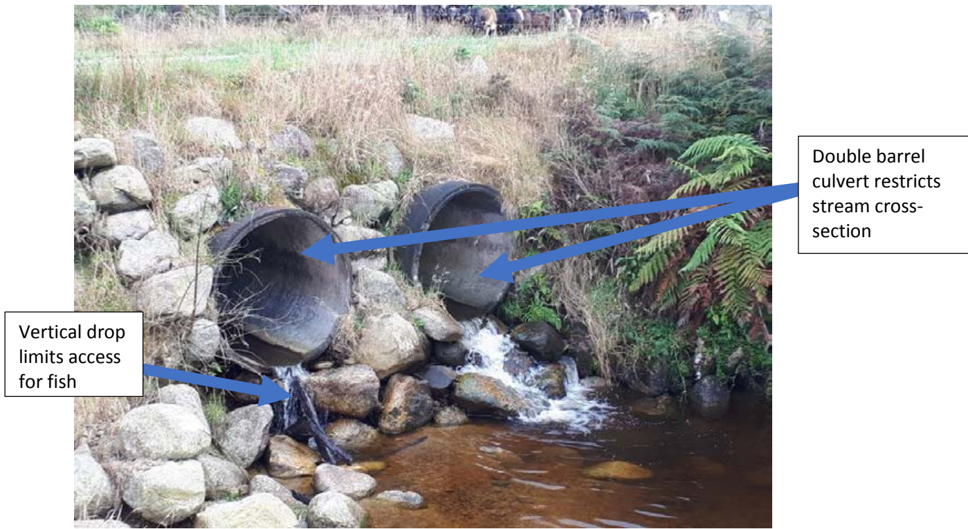
Figure E-16: A double barrel culvert where passage will be impeded by the fall height at the culvert outlet. Passage for climbing fish species may be possible over the rocks below the culvert in the right of the picture. Credit: Sam Ammon.
