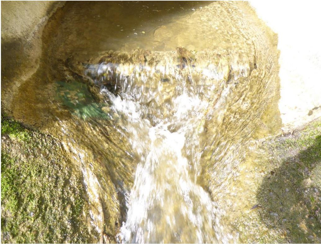
Figure I-6: Weir created by the baffle at the transition point between the culvert outlet and apron.
