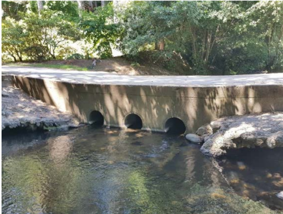
Figure 4-17: Raised roadway ford crossing with culverts. At low flows water passes through the culverts in the ford, rather than over the roadway. The small culverts used in this ford severely constrict the river channel and will result in accelerated water velocities through the culvert barrel that may be impassable to fish.
