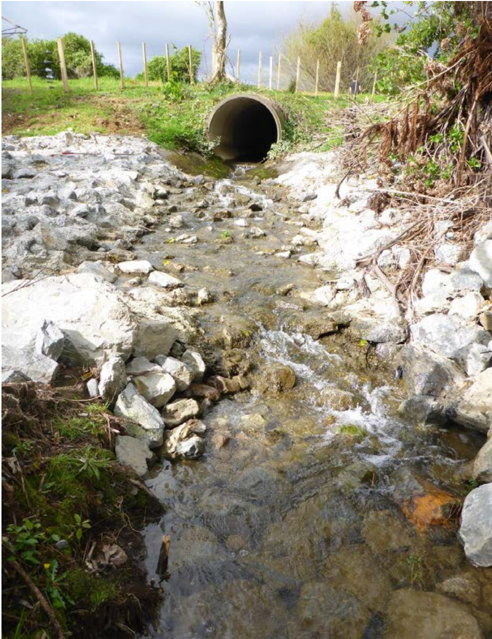
Figure 5-4: An example of a concrete rock ramp below a culvert in the Manawatu-Wanganui region. Concrete is used to prevent water seepage between rocks and is shaped to provide a low flow channel and resting pools to facilitate upstream passage. Photo: Cindy Baker.
