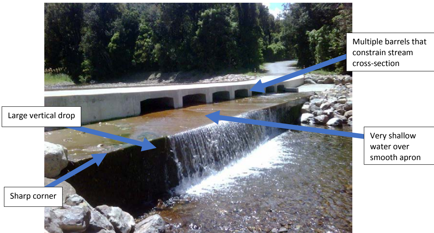
Figure E-18: An example of a drift-deck ford. This is a significant barrier to fish due to the large fall height on the downstream side of the structure. Passage may also be impeded by the sharp corner on the edge of the apron, shallow water, and high water velocities during high flow.
