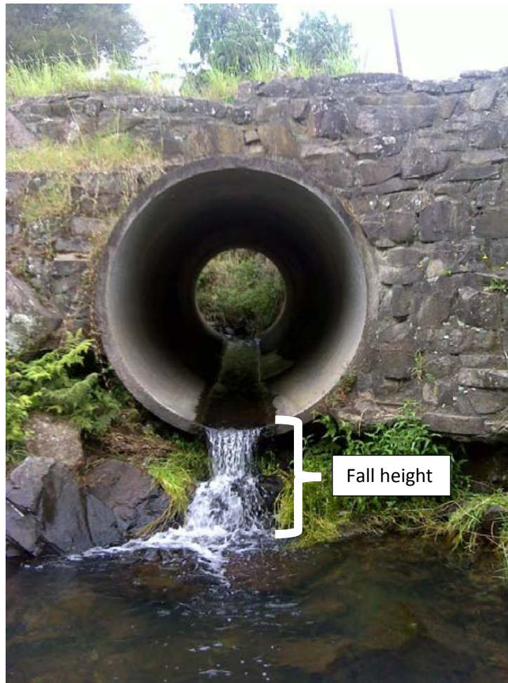
Figure E-1: Example of a perched culvert illustrating fall height.
