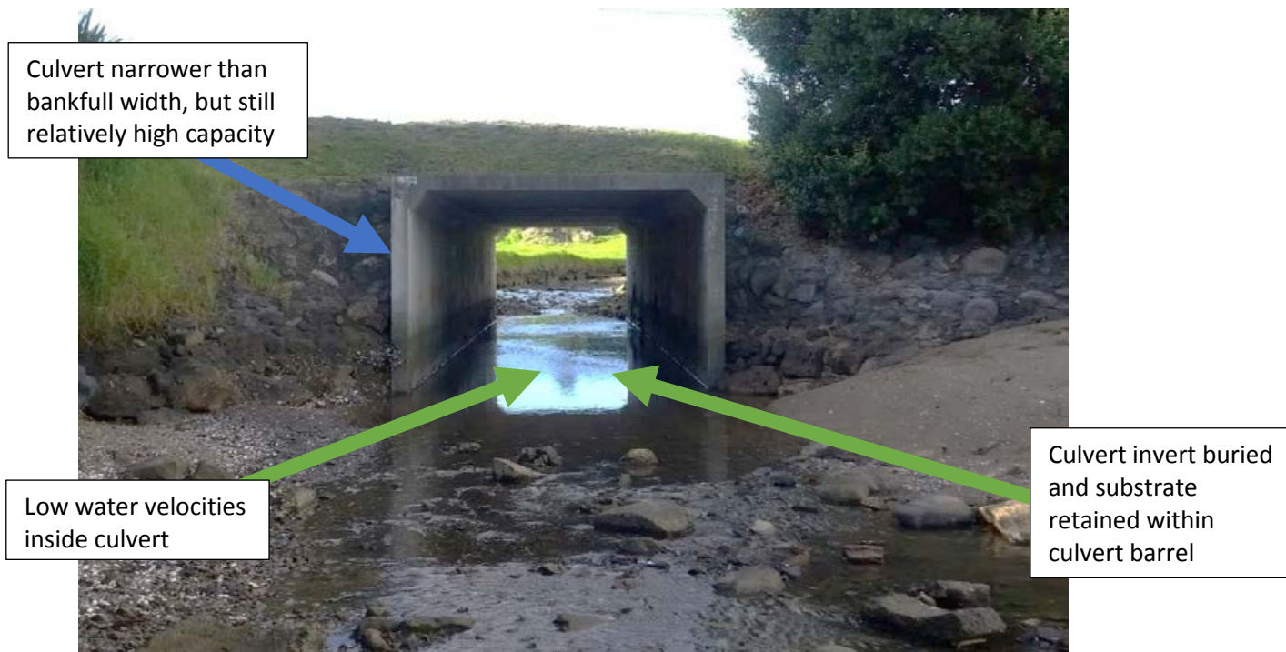
Figure E-22: Example of a culvert in a tidally influenced area. The culvert invert is embedded meaning that natural substrate is retained through the culvert. Culvert width relative to the stream bankfull width is lower than recommended, but because the culvert is in a tidal area, low water velocities will exist through the culvert during slack tide conditions. Credit: Bryn Quilter.
