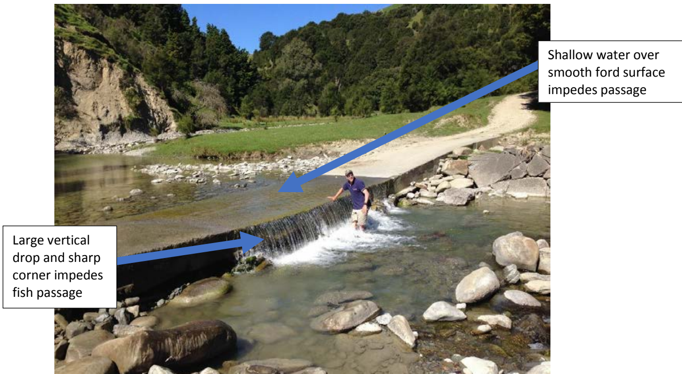
Figure E-21: The fall height on this ford on the Te Arai River is a significant impediment to the upstream passage of fish. Credit: Paul Franklin.
