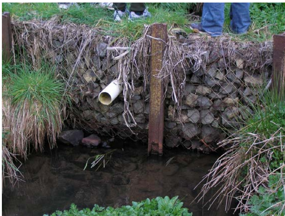
Figure 6-11: An unsuccessful gabion basket weir installed to allow migratory native fish access, while preventing trout access in Orokonui Creek, Otago. Credit: Sjaan Bowie.
