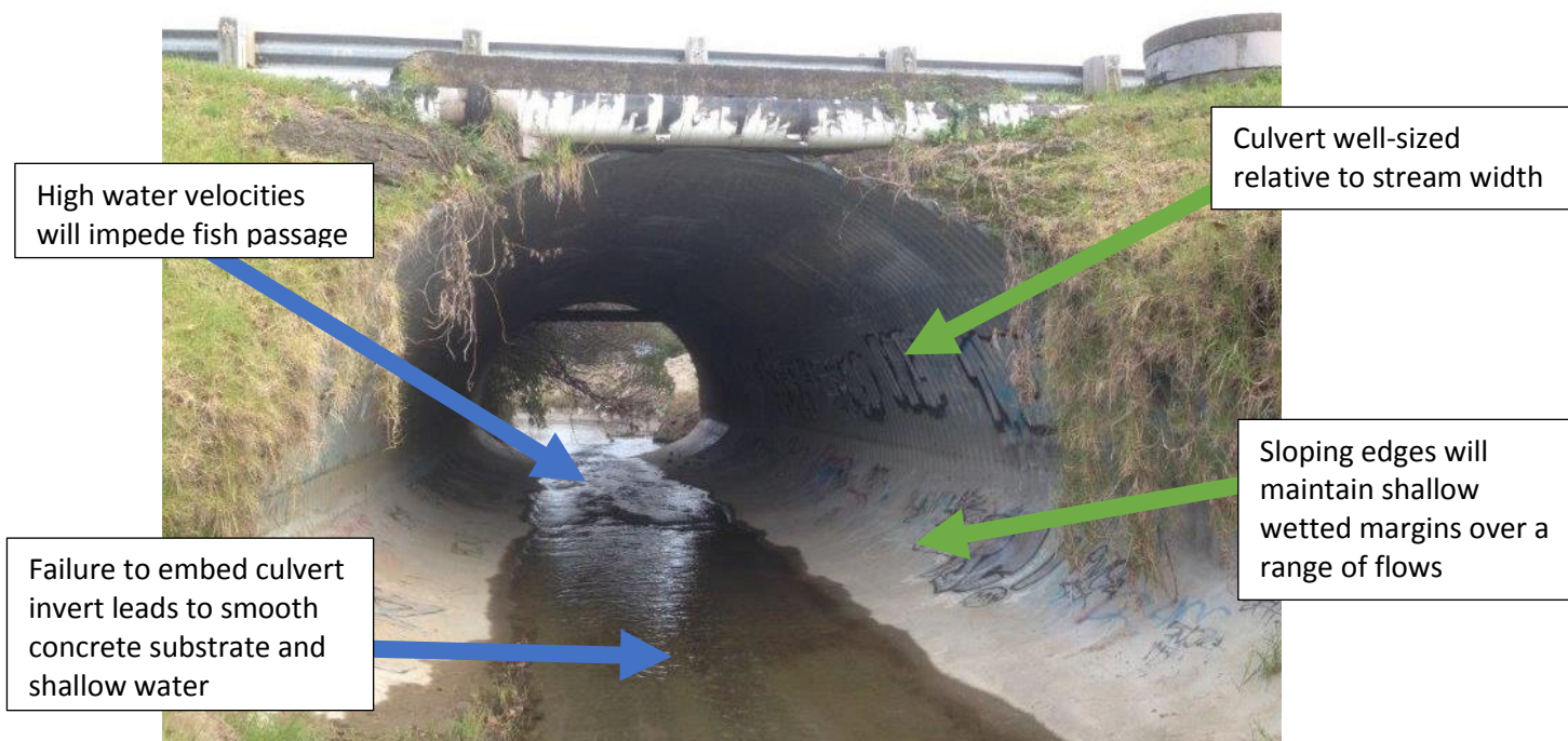
Figure E-23: Culvert well sized relative to stream width, but failure to embed the culvert invert leads to shallow water depths and high water velocity. If this culvert had been embedded so that substrate was retained through the culvert it would have been a good example of how culverts can provide fish passage. Credit: Mark Pennington.
