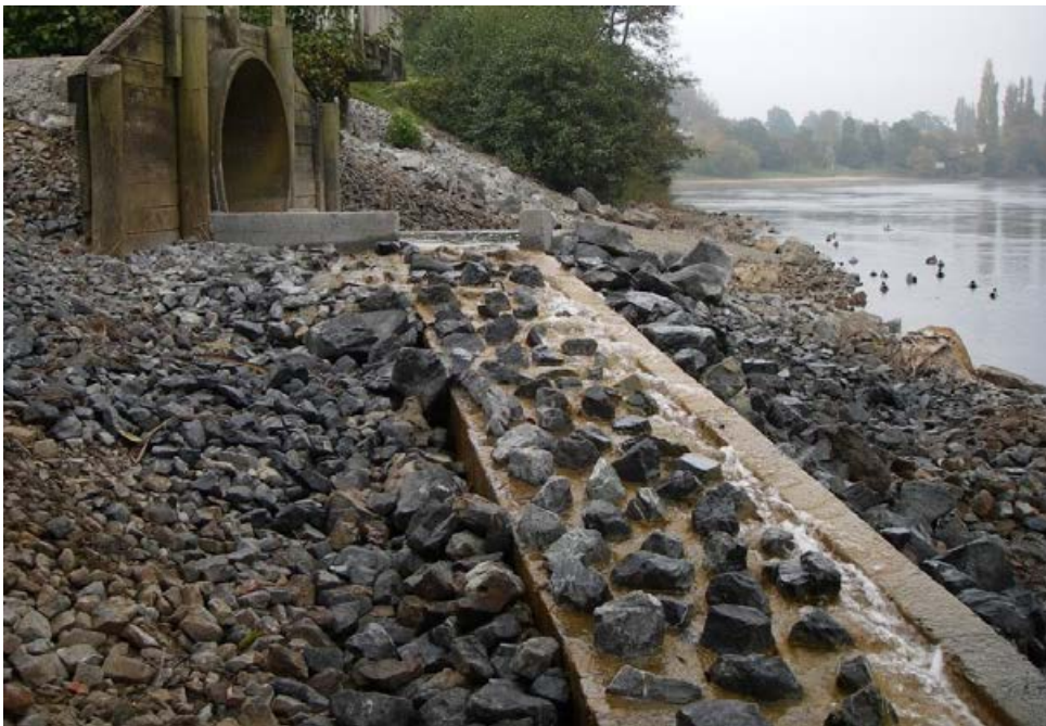
Figure I-14: The receiving pool and fish ramp operating under summer low flow conditions.
