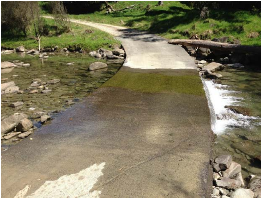
Figure 4-16: Raised roadway ford crossing. The vertical drop on the downstream side will block fish movements. Shallow water depth and elevated water velocities across the ford pavement can also impede movements.
