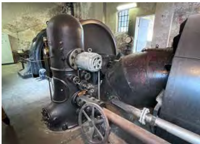
Eldre, hydraulisk (vanndrevet) regulator for turbin.
